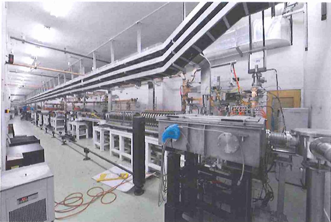
Overview of the SDUV-FEL Facility
